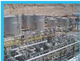
Co2 Plant - BAKU / AZERBAIJAN
