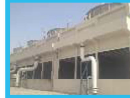
Cooling Towers - BAKU / AZERBAIJAN
