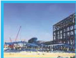
Brullus Power Plant 4800 MW PCESCO / EGYPT
